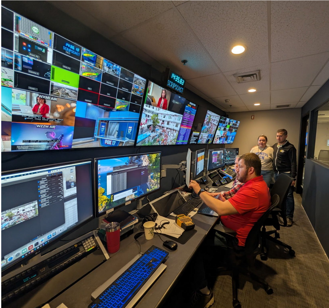
Control Room at WXMI, Grand Rapids, Michigan
